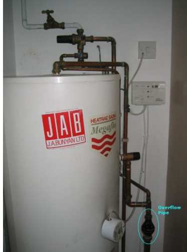
Radiant Winterization Boiler
