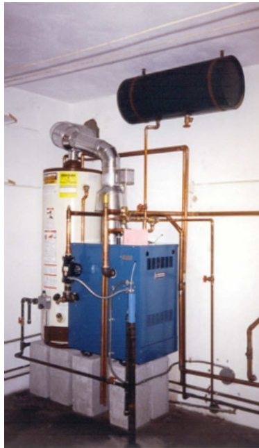
Radiant Winterization Expansion Tank
