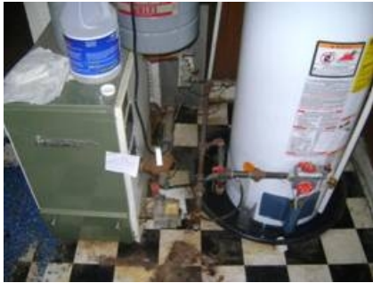
Steam Winterization Boiler
